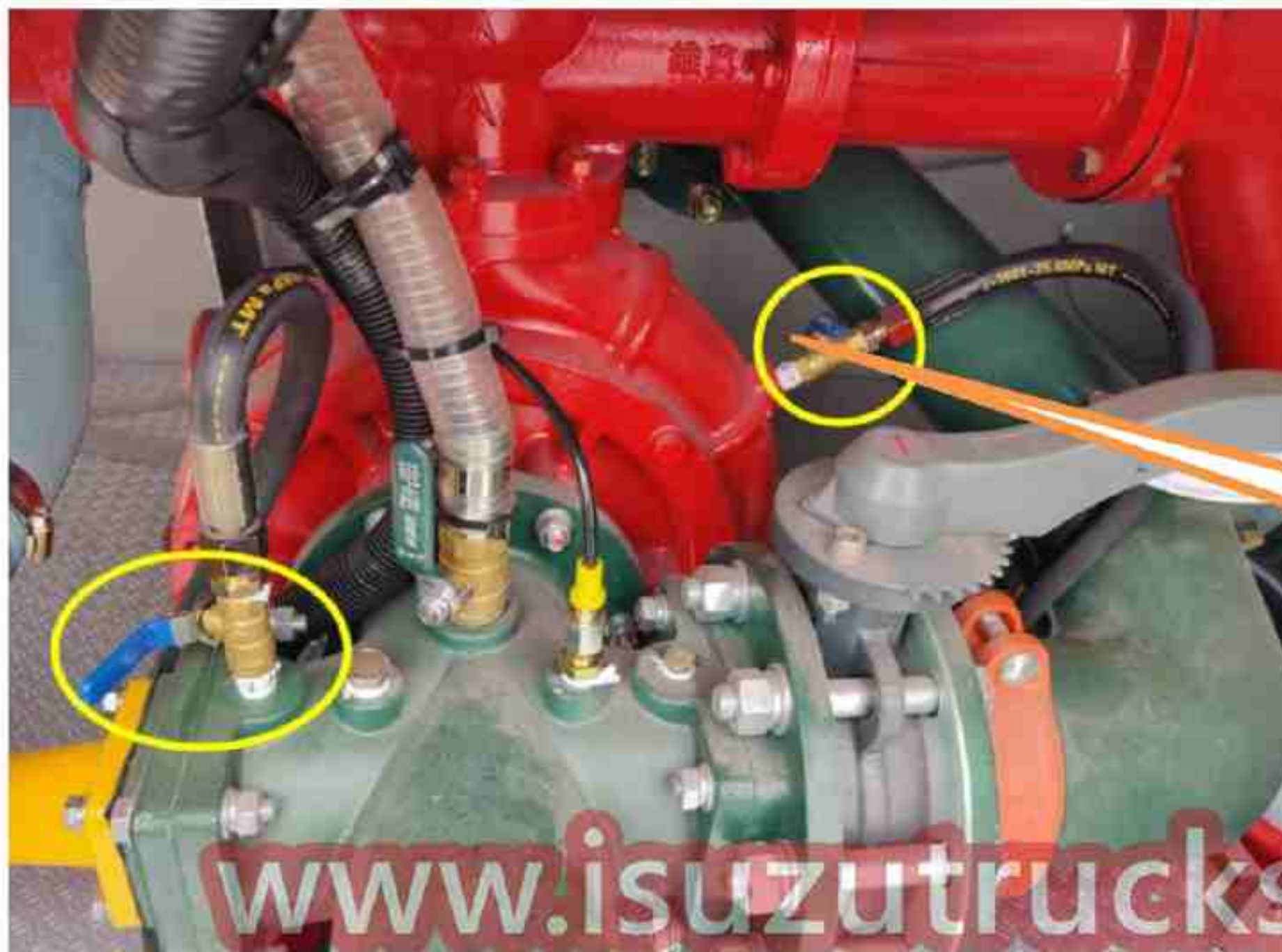
Inlet and Outlet valve for cooling system
